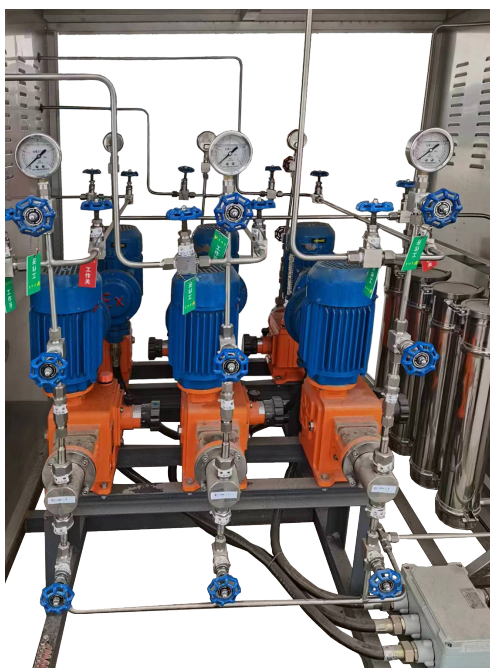
Process Chemical Injection Skid
