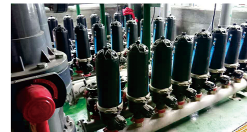
Membrane System Protection Filtration
