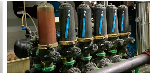
Wastewater Treatment Plant Water System Filtration
