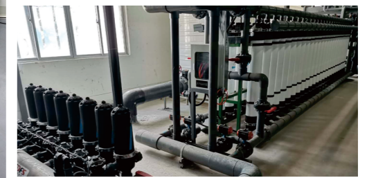
Membrane System Protection Filtration
