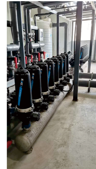
Hvac Water System Filtration
