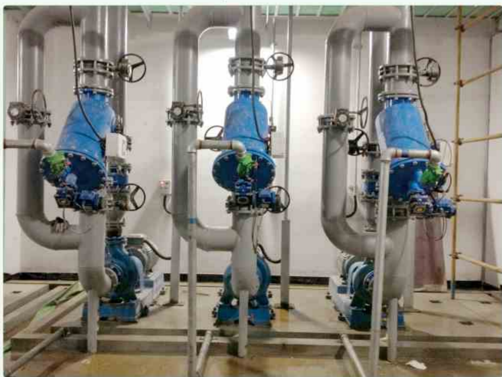
Power plant cooling water filtration
