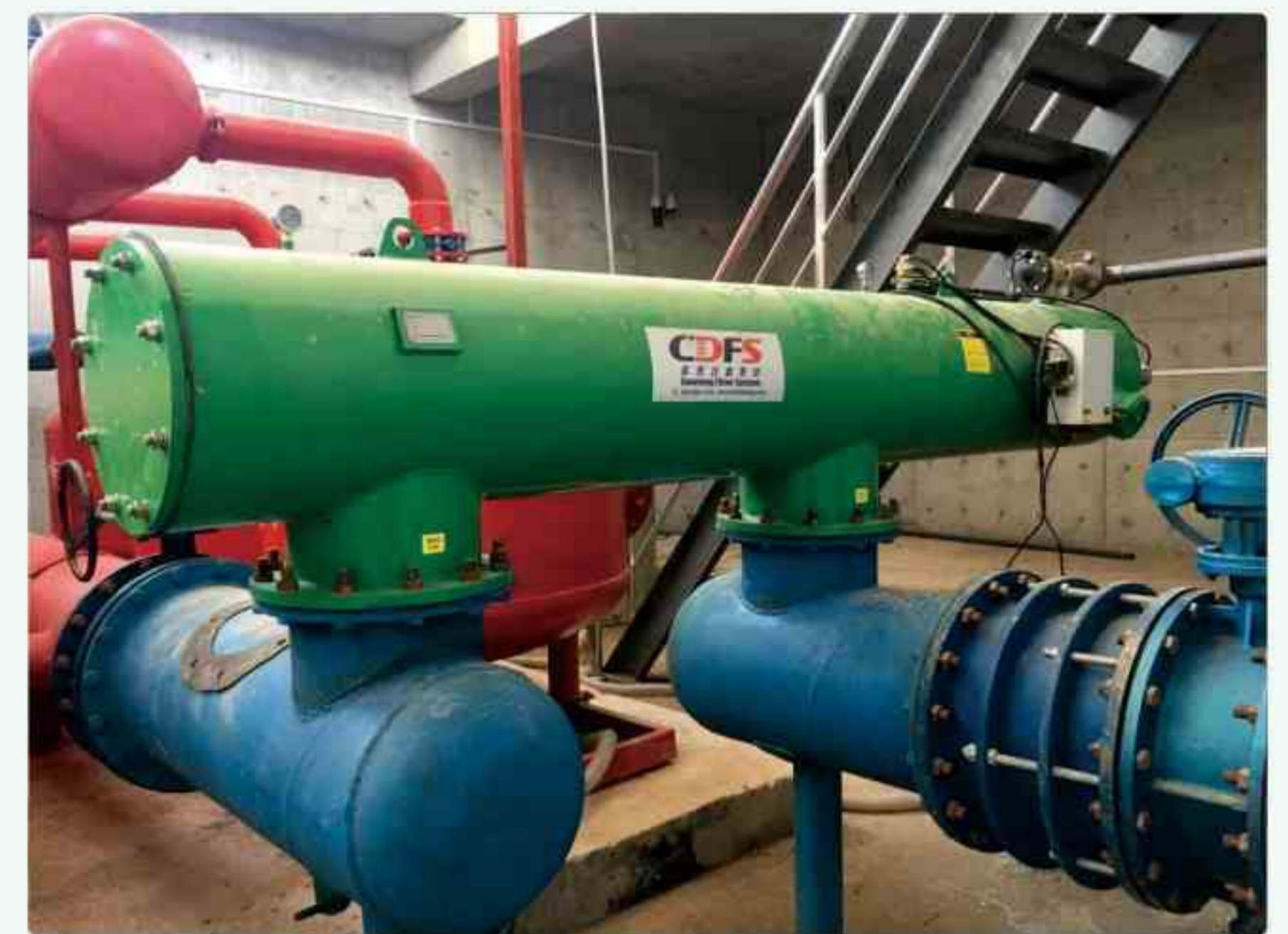
Filtration for irrigation
