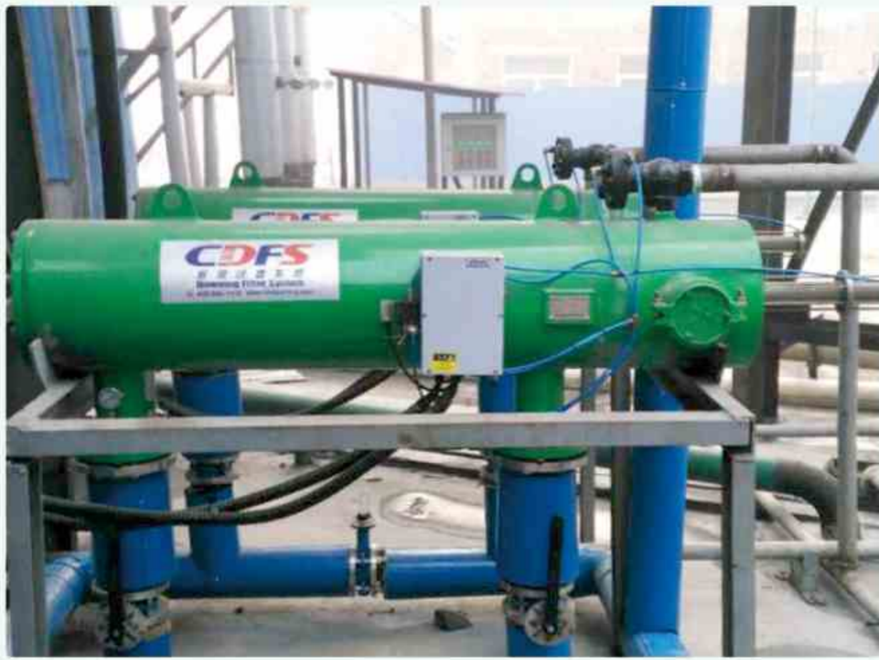
Desulphurization wastewater filtration
