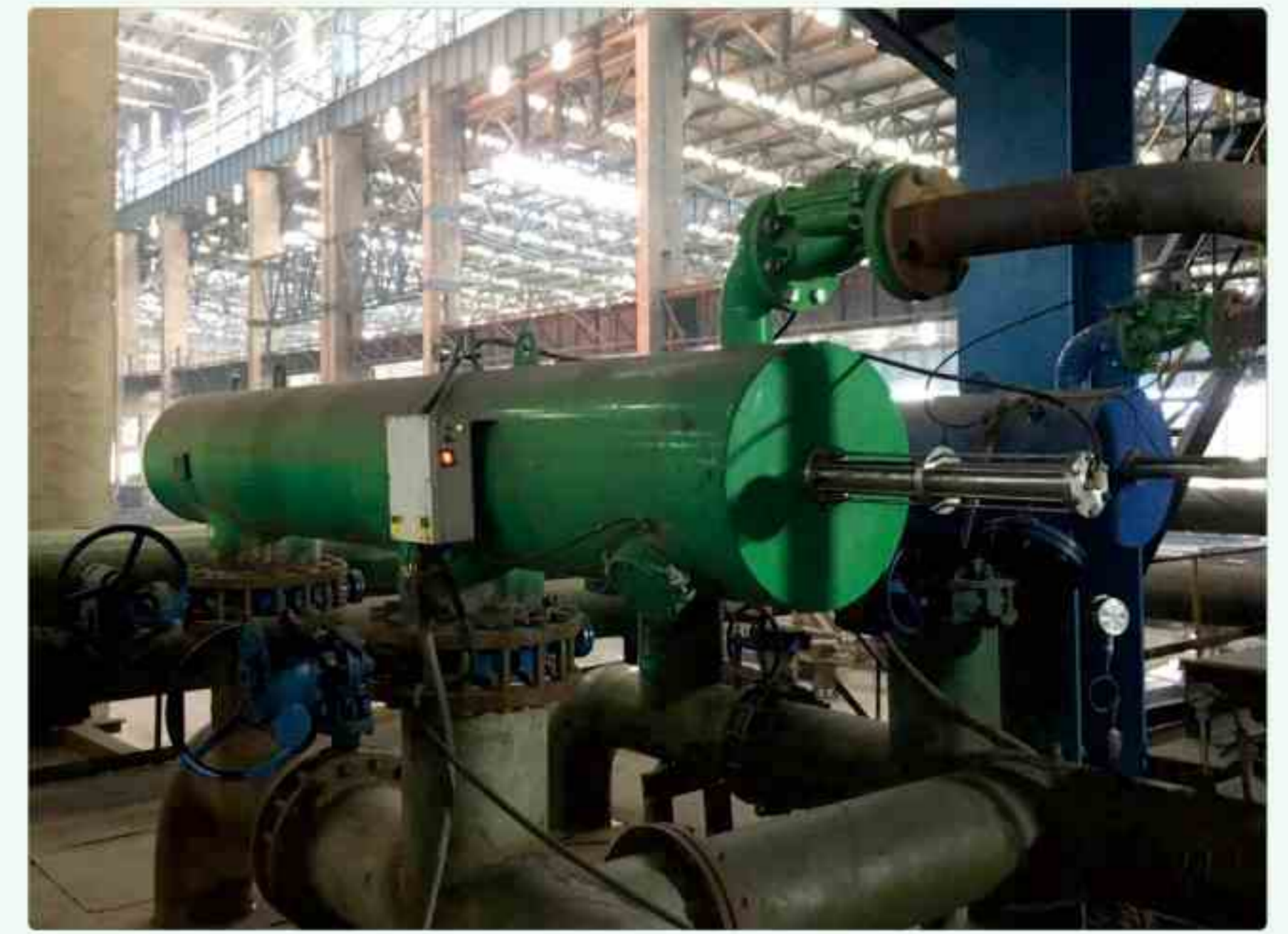
Cooling water filtration of copper iron plant
