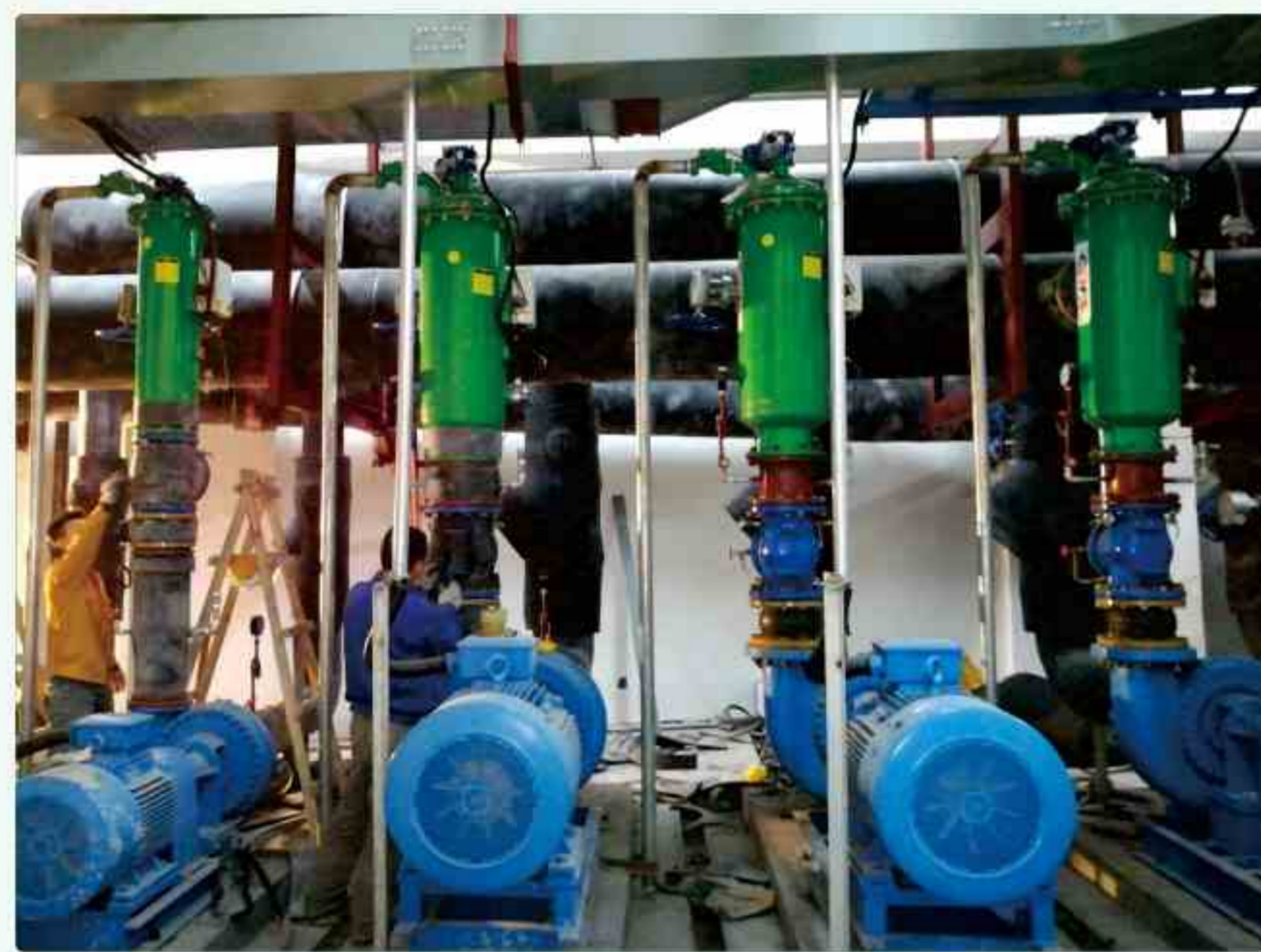
Cooling water filtration of buildings
