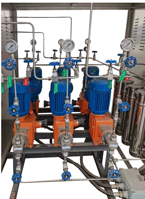
Process Chemical Injection Skid
